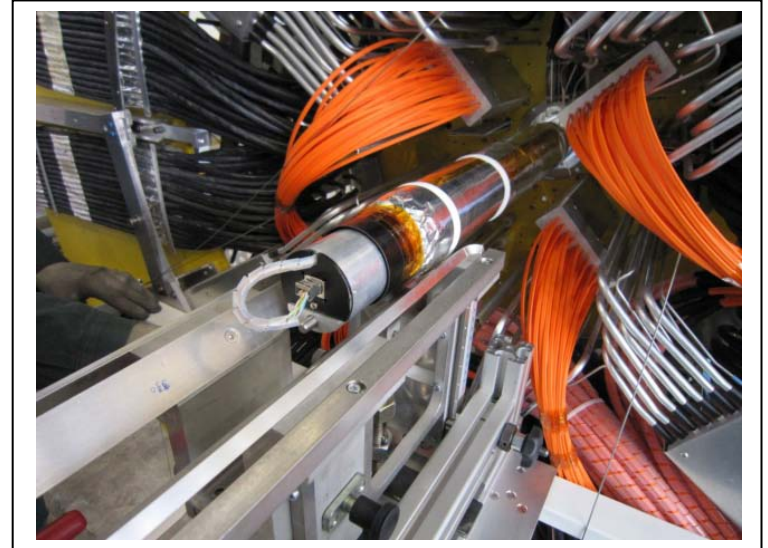
LGT supporting BP0 on side C
